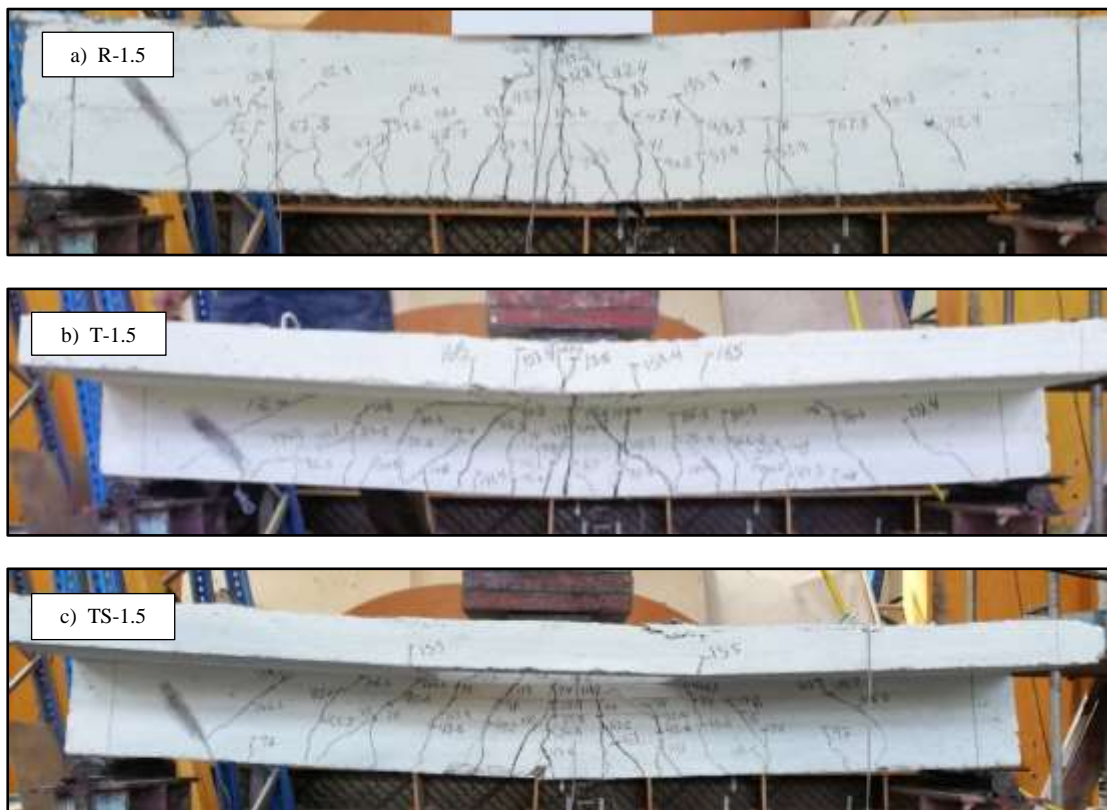
Fig.3 Crack Pattern of Tested beams
