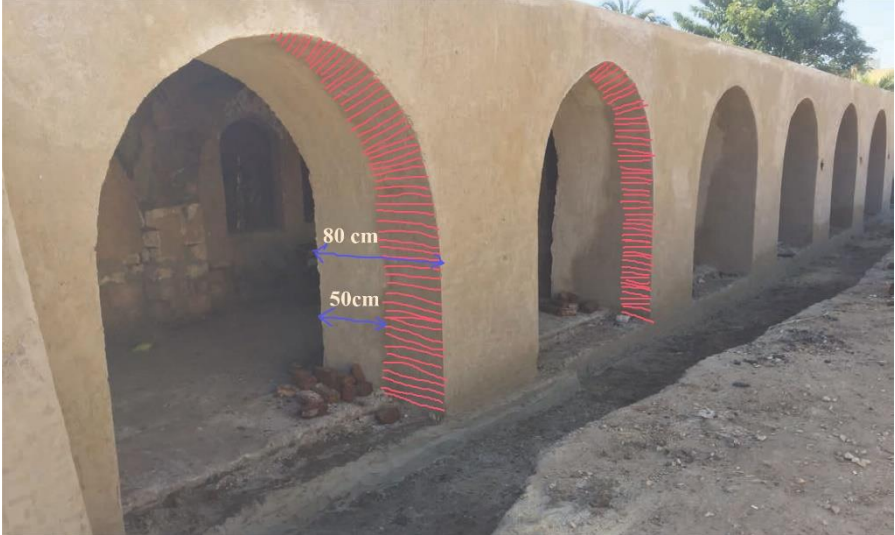
D: During and after applying the clay plaster to the northern facade wall.
