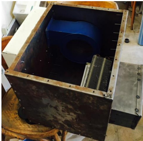
(a) AHU from inside
