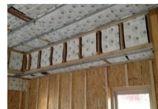
Fig. 22. PCM integrated in ceiling [44]
